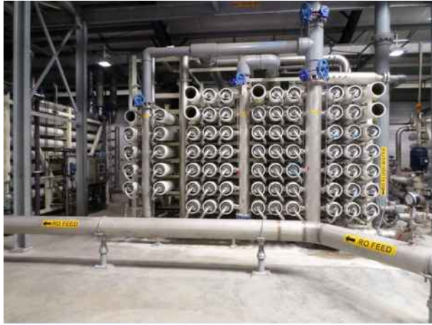
Existing RO System
